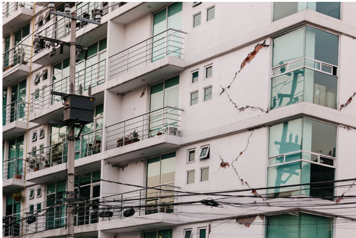
Earthquake damage on an apartment building in Mexico City.
